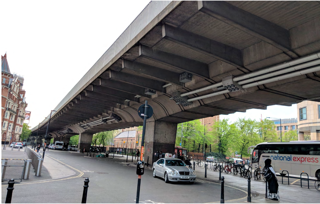
Figure 5. Replacement post-tensioning system on Hammersmith Flyover showing the external “short” tendons anchored by UHPFRC blisters.
